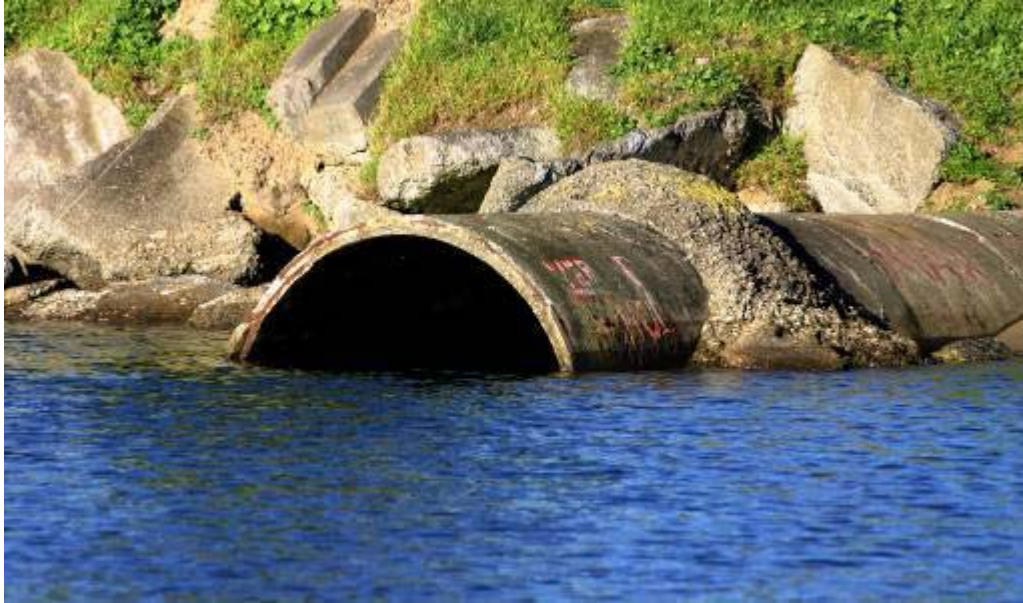
Figure 2.1: Stormwater outfall at Evans Bay in Wellington City – diluted raw sewage can be discharged with stormwater from this outfall during times of heavy rainfall
