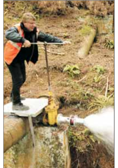
Mark Poehls, operations foreman, flushes a water main near Porirua. Greater Wellington collects, treats and delivers about 150 million litres of water each day to the four cities in the region. Maintaining the water supply system is essential to ensure the reliable delivery of high quality water.
