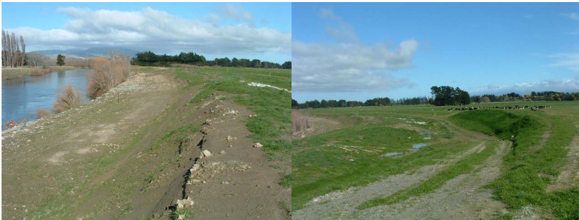
Picture 3: riverside berm to be lowered (left); extended stopbank and realigned sill (right)
