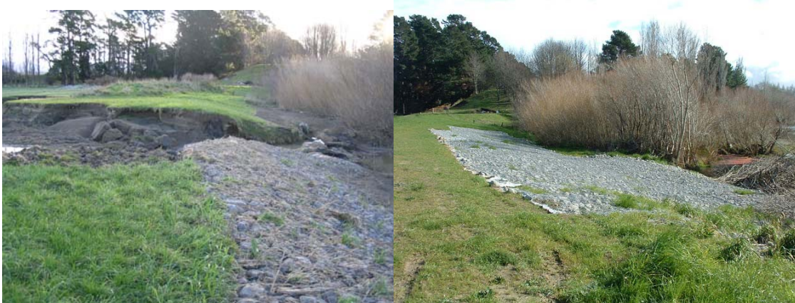
Picture 2: damaged 'Duckbill' drop structure (left) and the repaired structure (right).
