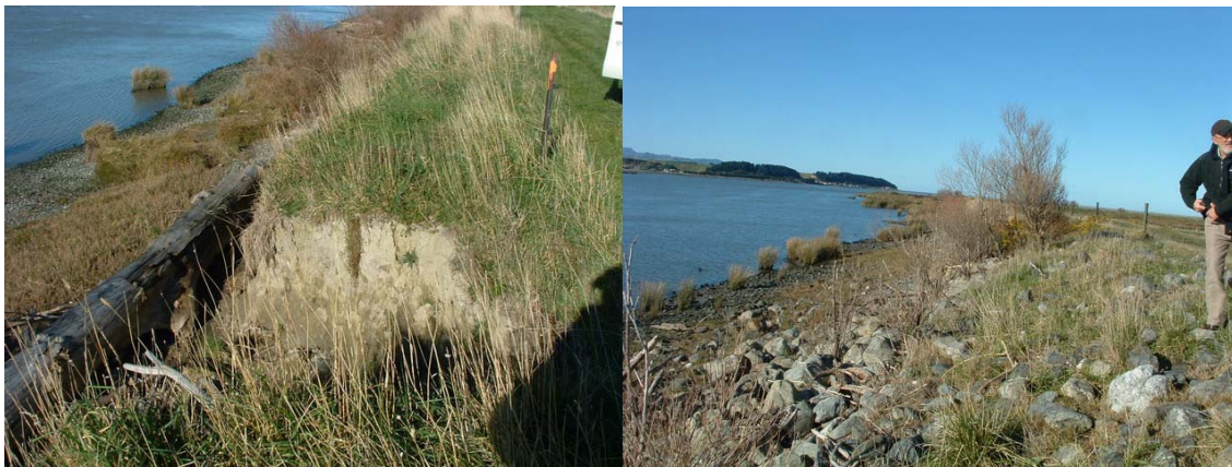
Picture 1: erosion 'hole' (left); repaired stopbank (right)
