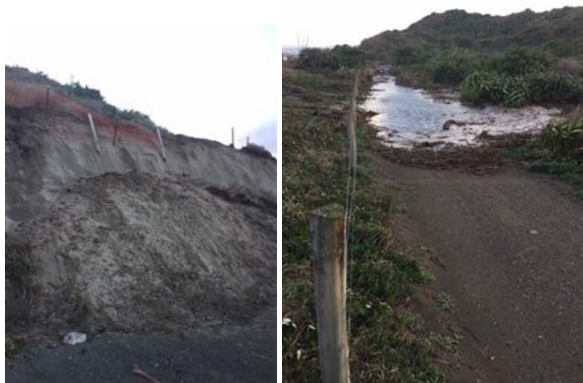
Coastal track damage showing a) dune undercutting and b) inundation of a section of the track.
