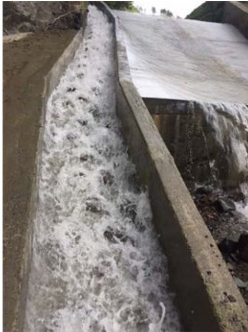
Woollen Mills Dam – showing the new fish pass (left) and resurfaced spillway (right).
