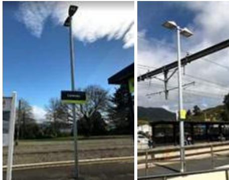
Figure 45: Shelter lights at Redwood Station
