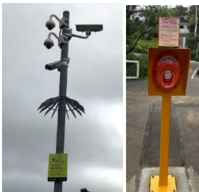
Figure 43: Station CCTV cameras and duress help point
