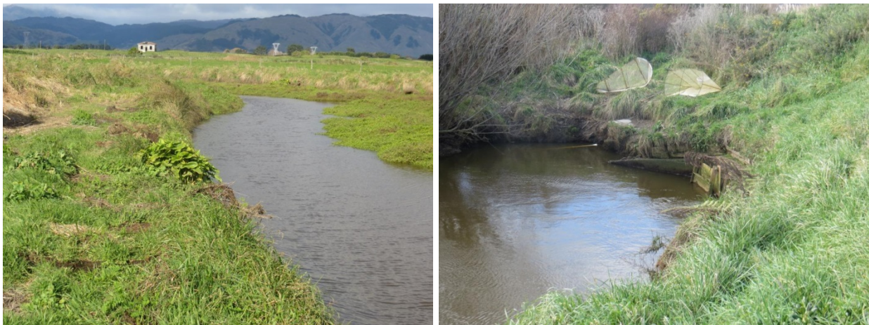
Figure 3-5: View of Pahiko Drain (left) and culvert through stopbank at Otaki Estuary (right)
