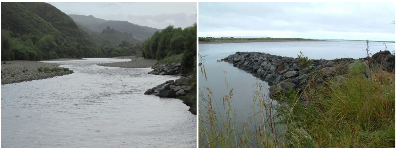
Figure 5-1: Rock groynes, Hutt River (left) and a large rock groyne near Otaki River mouth (right)
