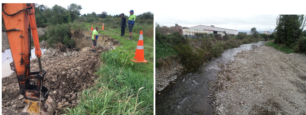
Photos of repairs on the Mangatarere River to CDC wastewater pipe (left) and strengthen vegetation on the Waipoua River right).
