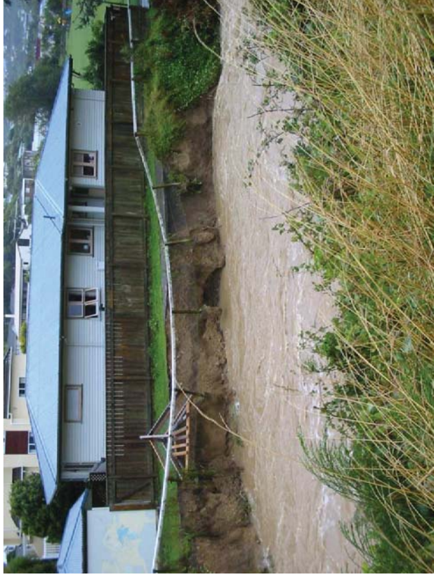
Porirua Stream 13 Tawa St. Erosion 16 Feb. 04
