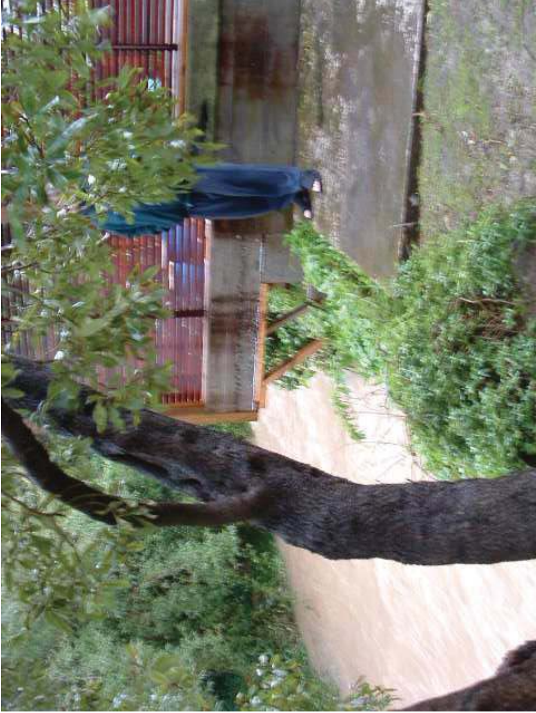
Deck 24 Oxford Street over Porirua Stream 17 Feb 04 – 7 yr return period flood event on the Porirua Stream
