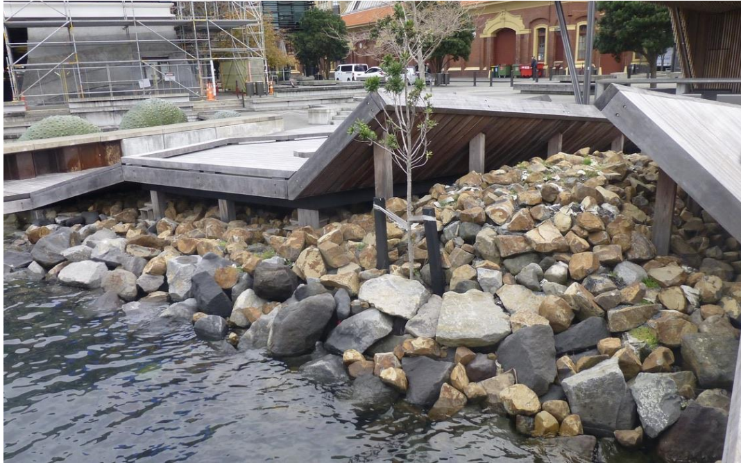
1 A portion of the northern rip-rap, with new rock laid over old rock. Kumutoto North park beyond.
