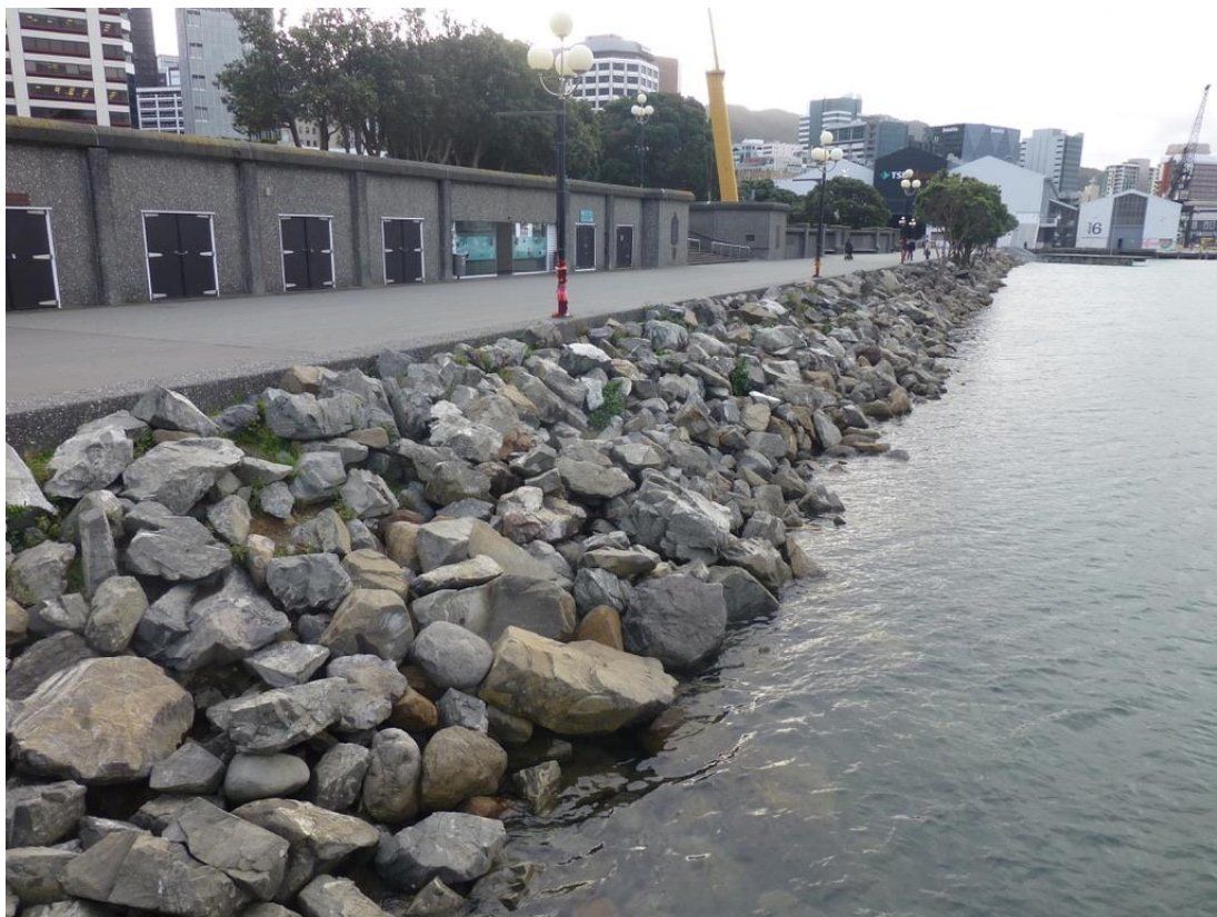
4 The southern section of the rip-rap looking north towards Queen's Wharf. Frank Kitts Park on the left and Shed 6 in the distance.
