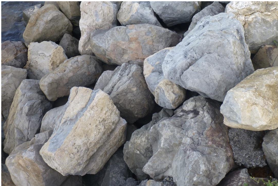
6 Detail of the rocks of the southern section of the rip-rap. All photos, June 2020.
