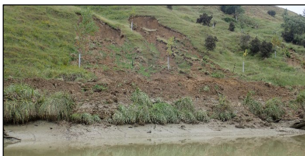
Land slip on steep estuary margin after heavy rainfall, and turbid water column
