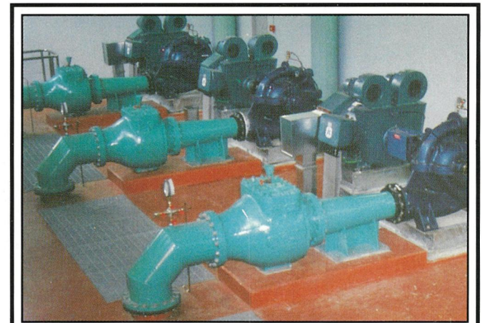
Water Pumps and Motors
