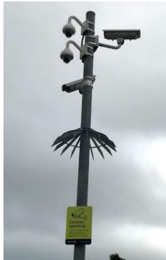
Figure 44: Station CCTV cameras
